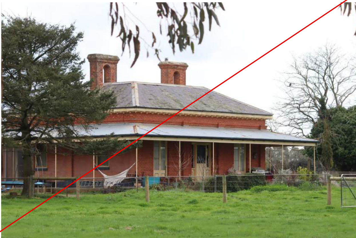
Close-up of the façade (right) and south elevation of Bernera Homestead. Note that the slate roof tiles have been lost. (Source: RBA, August 2024)
