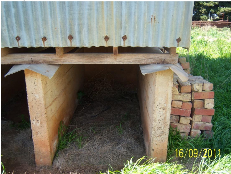
Plate 12: Side base view of Nissen Hut in a farm on Ferris Road utilised for grain storage (Photograph courtesy of S.J. Peters, 16.09.2011).
