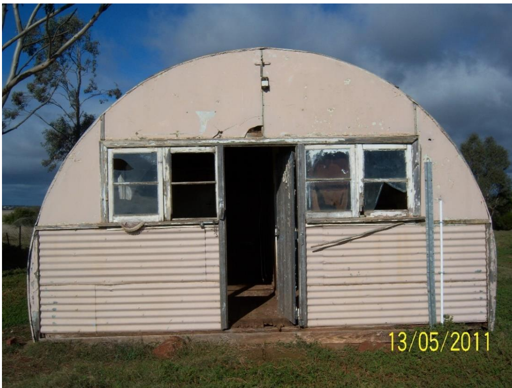
Plate 16: Front view of Nissen Hut along Bridge Road Melton South (Photograph courtesy of S.J. Peters, 13.05.2011)
