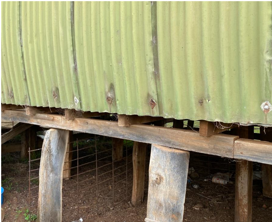
Plate 4: Detail showing the fastenings used in the hut's construction (Photograph by M. Filihia 12.05.2022)
