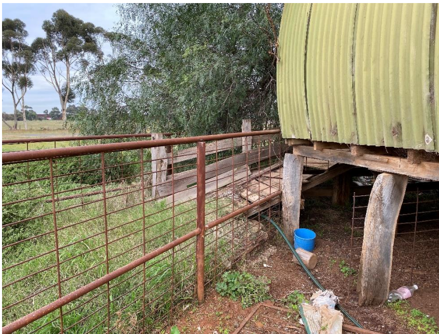
Plate 9: Study area facing south-west showing stockyards made from a variety of fencing. Note the timber ramp with loose planks into the Nissen hut (Photograph by M. Filihia 12.05.2022).
