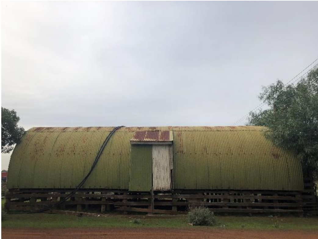
Plate 2: Study area facing east showing Nissen Hut at 1232-1290 Beattys Road (Photograph by G. Polic 12.05.2022)
