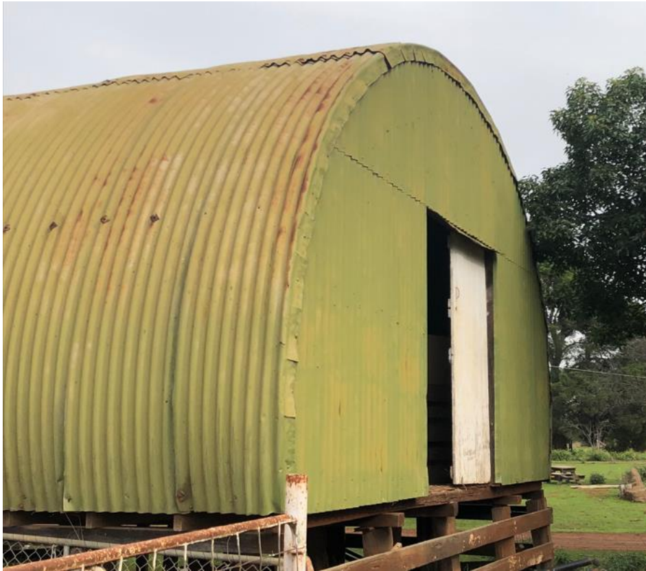
Plate 5: Study area facing south-west showing the double door on the northern elevation of the Nissen hut (Photograph by M. Filihia 12.05.2022).
