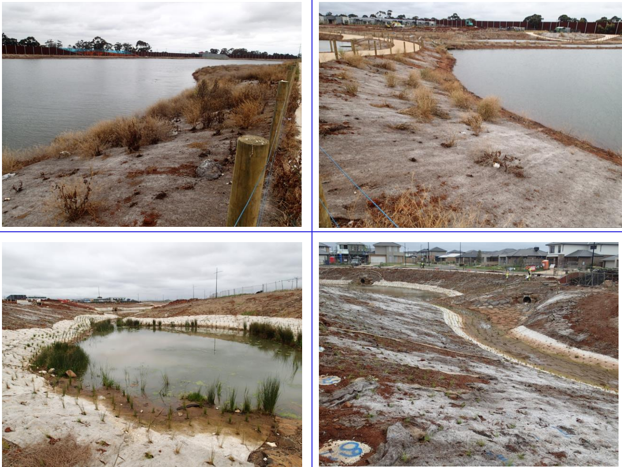
Figure 5-2. Constructed retardation basin near Western Freeway in Paynes Road Precinct/Shogaki Drive DSS (Top left and right) and connecting waterway corridor (Bottom left and right). Batter treatments comprised of geofabric with direct planting into underlying clay soils. Rock work is evident within the vicinity of drainage outfalls. Photos dated 4 October 2022.
