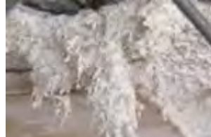
Loose fibres - friable
