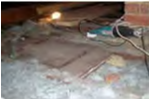
Friable asbestos debris (friable)
