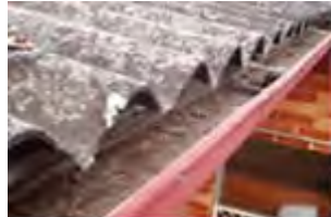
AC moulding gutter (friable)
