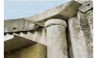
AC downpipe (friable)
