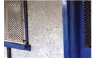
Chrysotile pebble dash exterior wall coating (non-friable)
