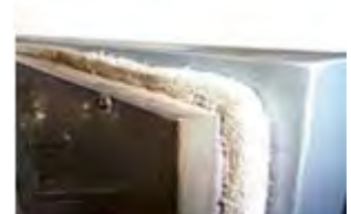
Asbestos rope seal on drying oven (non-friable)
