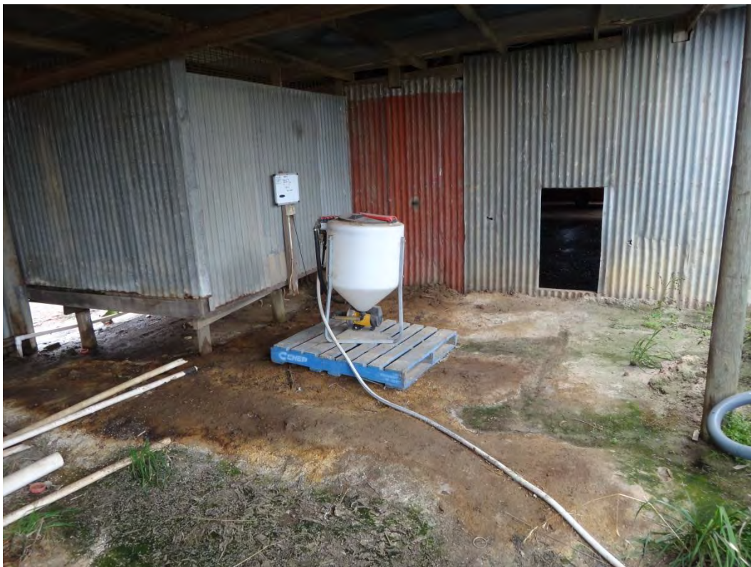
Photograph 138: Chemical (herbicide etc...) mixing pump located in the north portion of the property behind the storage/processing shed.
