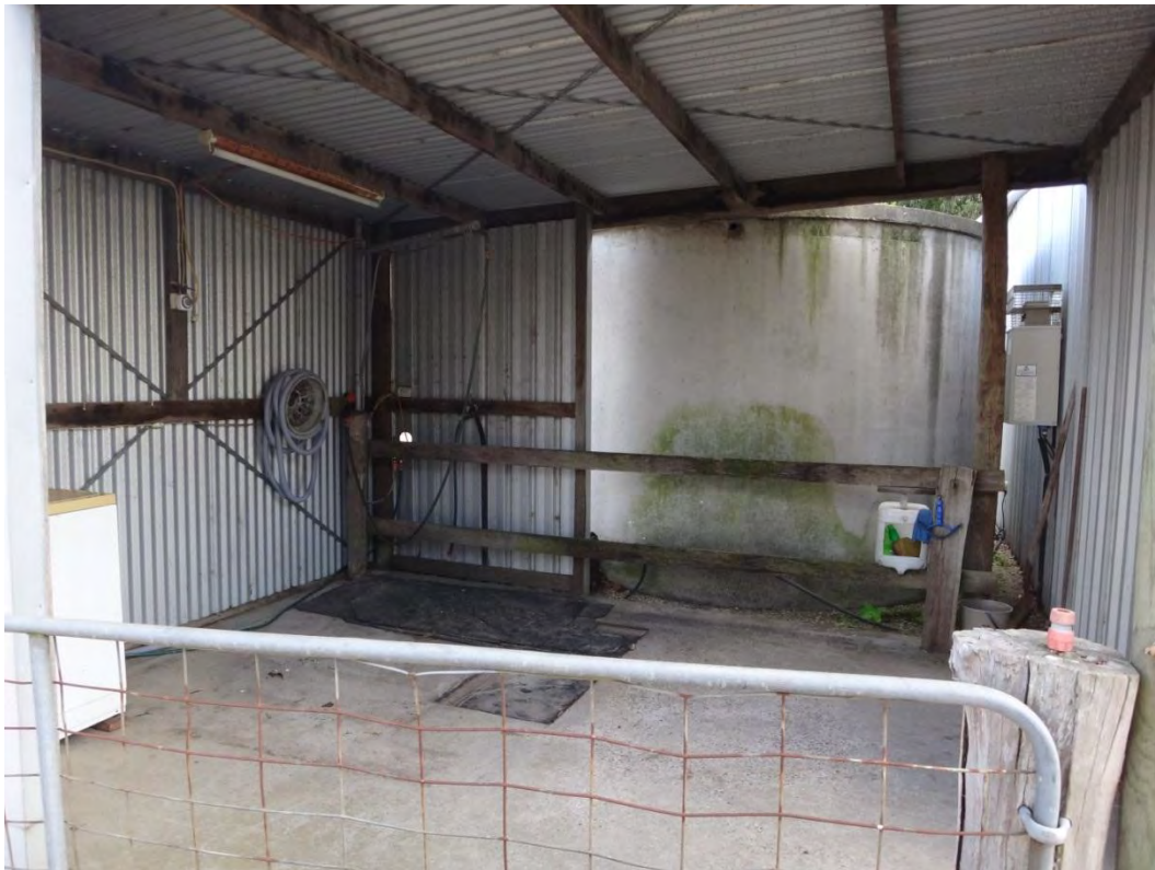
Photograph 69: Animal wash down and cleaning pad.
