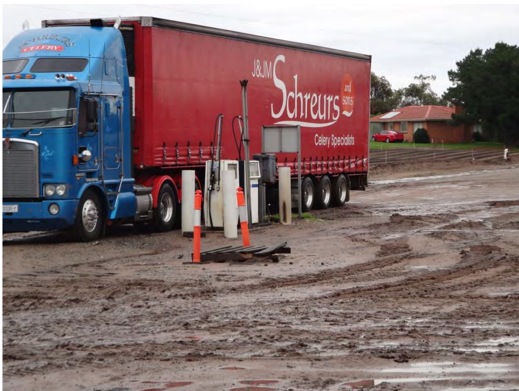
Photograph 134: Refuelling bowsers linked to diesel USTs.
