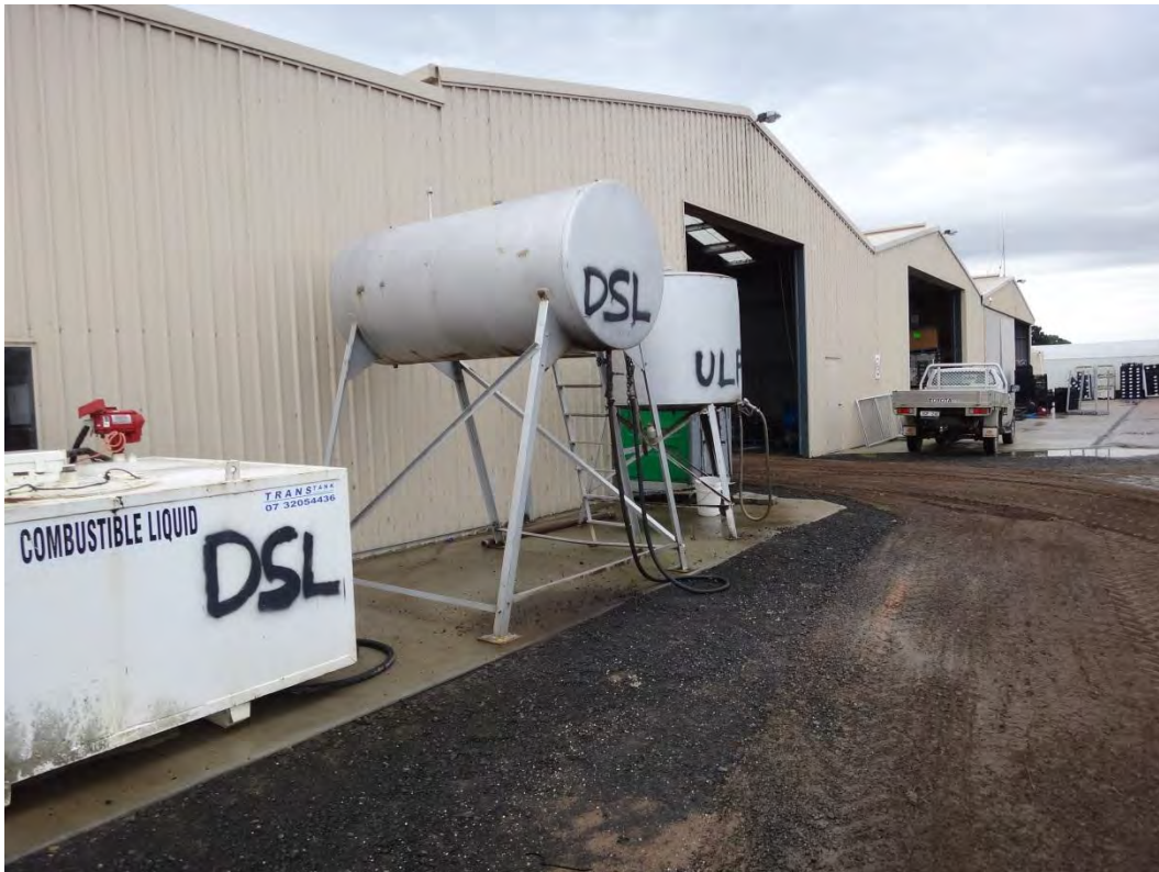
Photograph 150: Diesel and unleaded fuel ASTs located to the north of the processing and maintenance shed.
