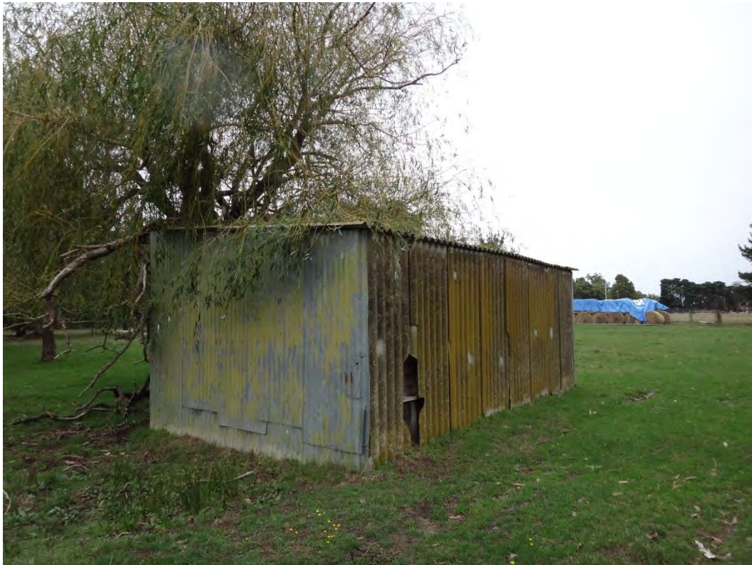
Photograph 144: Former stock shelter potential asbestos cement wall.
