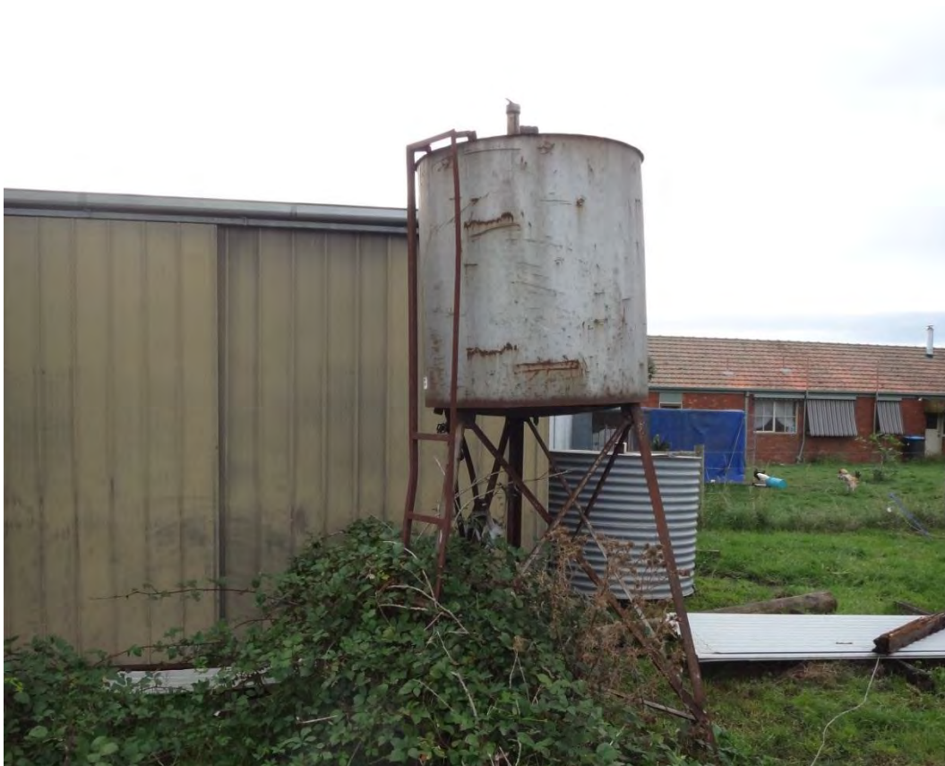
Photograph 2: Diesel AST adjacent to the rear (west) wall of the garage and residence.
